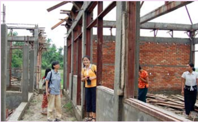
Cathy and Usha visit an under-construction school they helped to raise funds for
